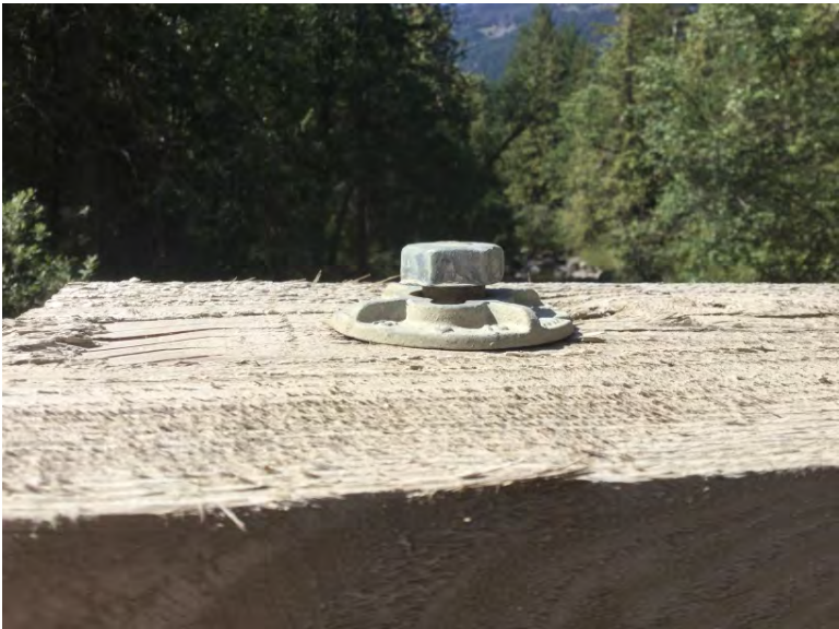
Loose hardware on rail, typical
